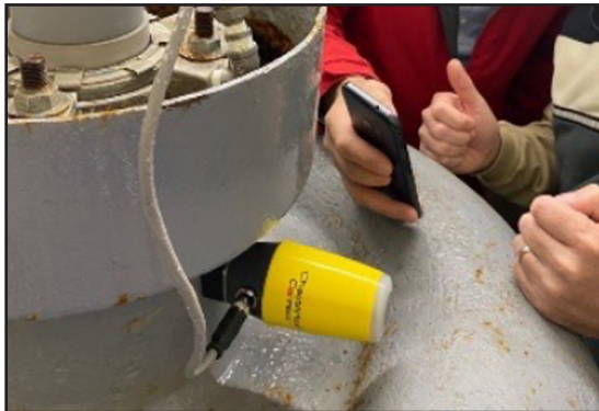
Chesterton Connect Sensor installed on the pump.
